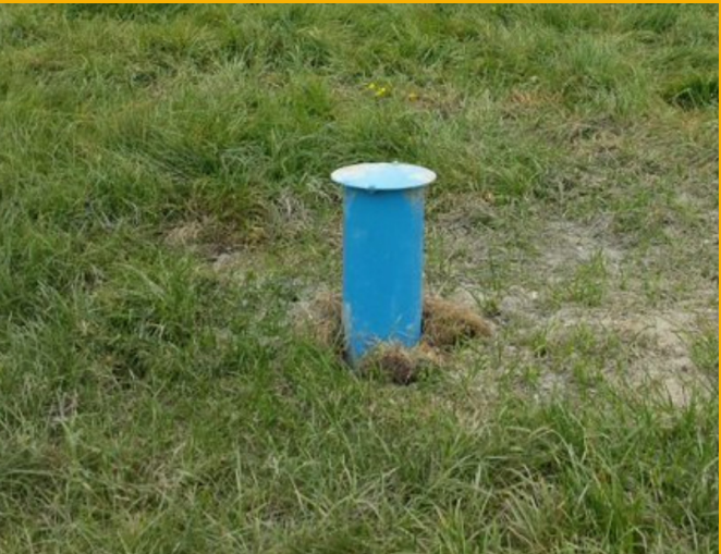
Examples of a raised borehole cover
